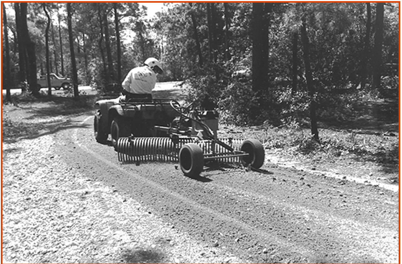
Figure 14—The trail rake and Ultra Light Terrain Grader worked great on campground roads and parking lots.
