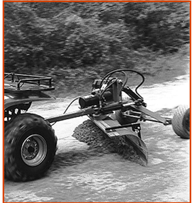
Figure 5—With two passes, the trail rake could pull in berm material from both sides to the center of the trail or road. Here, the scraping blade is being used.
