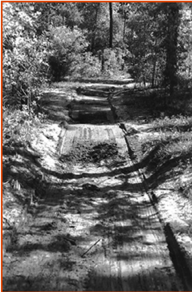
Figure 1—Evaluating equipment that effectively cuts the mounds and fills the depressions on washboard trails is what this report is about. This trail has been partly graded to remove the whoop-de-dooos.
