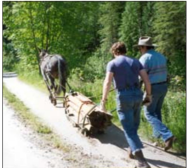
Figure 33—Fremont grader being used to haul waterbar materials. The grader blade has been removed.
