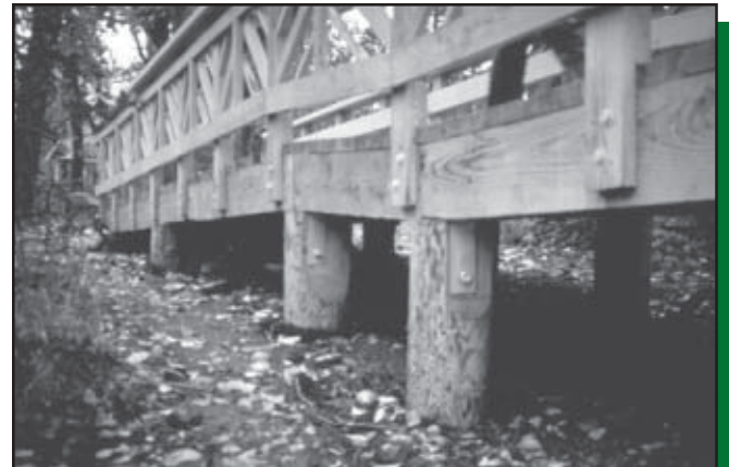
Figure 52—A typical boardwalk. Boardwalks are expensive and somewhat complicated, so seek the help of engineers and landscape designers during planning.
