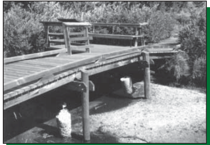
Figure 44—Know your soil conditions. Concrete end-bearing piles settled 1 to 2 feet here, and had to be replaced with these log friction piles.
