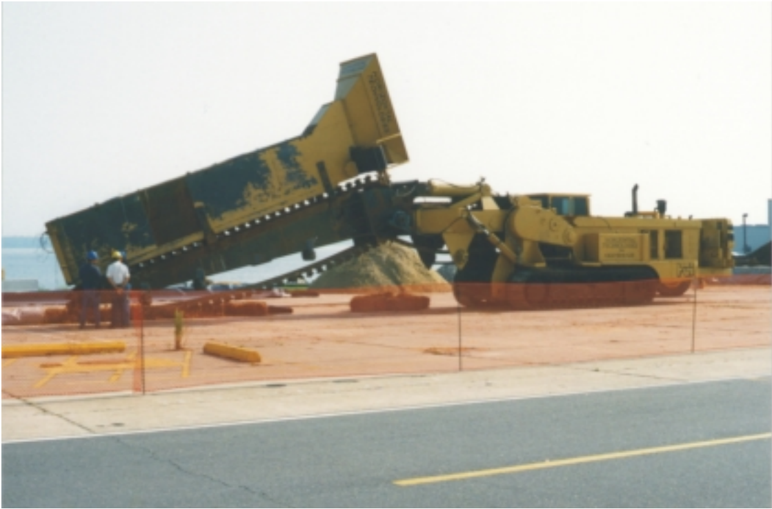
Figure 55. Trenching machine used to install the 7.3 m deep, 0.6 m wide granular iron barrier.
