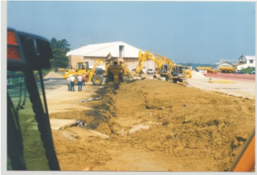
Figure 57. Picture showing collapse of concrete pavement on either side of the trench.
