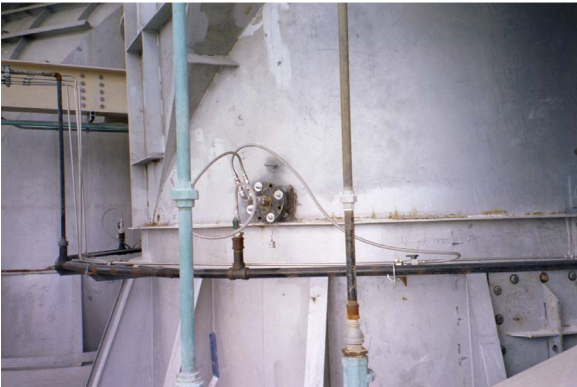
Figure 8-7. SNCR injection location – Suwannee American Cement, Branford, Florida.
