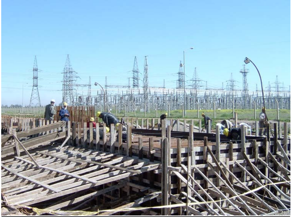
Photograph of the construction of the platform for one of the electric generation plants. (Photograph was taken on March 9, 2004.)
