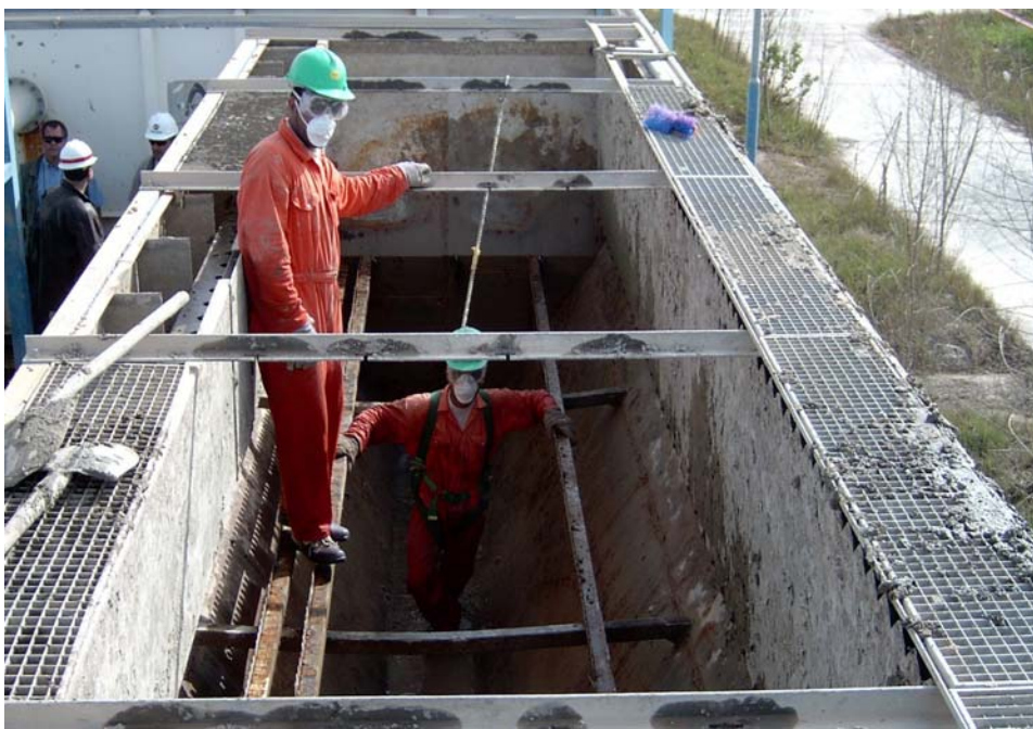
Photograph of the cleaning of one of the water filtration treatment units. (Photograph was taken on February 23, 2004.)
