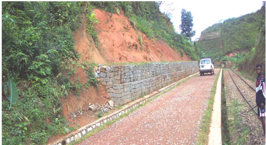
Photograph of the same portion of Road RNT14, with railroad, showing the repair and rehabilitation work conducted by the Mission. (Photo by contractor personnel, August 2002)
