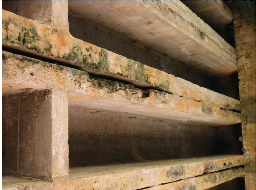
Figure 2 – Photograph of concrete beams with corroded steel strands and filtered-down moisture below Los Achiotes bridge in Olancho, Honduras, September 2003
