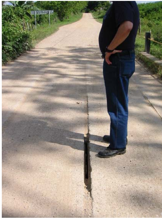
Figure 3 - Photograph of separated concrete slabs on the deck of Zopilote bridge in Olancho, Honduras, September 2003
