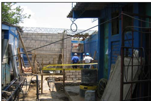
Photograph taken in March 2004 of an Office of Inspector General auditor and project personnel inspecting a reconstruction project site near Sonsonate, El Salvador.
