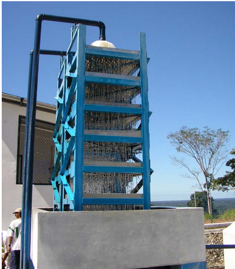
Photograph of Cascales water aeration tower taken in June 2004.
