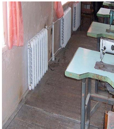
Photograph of an Armenian school's new heating system provided under the Heat Assisted Education Project, March 2007.
