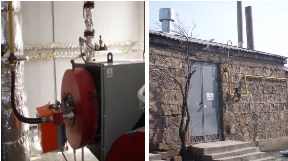
Photograph of a gas boiler installed in a maternity hospital in Yerevan, Armenia, as part of the Armenian Energy Assistance Project, March 2007.
