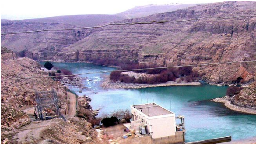
OIG photograph from atop the Kajakai Dam looking down at the power plant. (January 2007)
