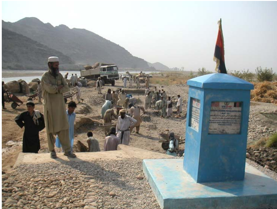
OIG photograph of Afghan men working on a cash-for-work project to build a flood protection wall for the village of Binigah. (October 2006)
