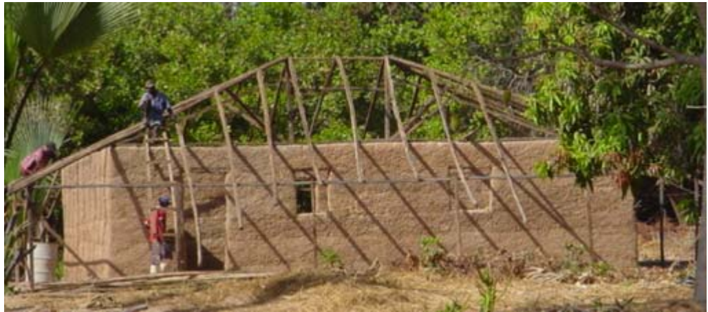
Photograph of a home being reconstructed with the help of Catholic Relief Services and USAID/Senegal in the Madina Mancagne village. (Photo taken February 5, 2003)
