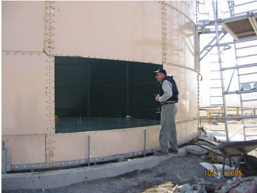
Photograph taken on October 11, 2005 by an OIG auditor of the water reservoir under construction.
