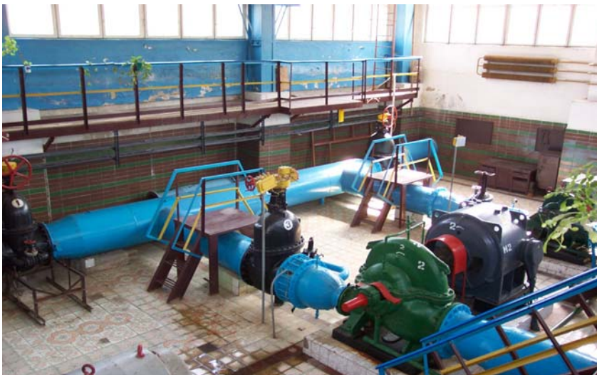
Photograph taken April 10, 2006 of a water pumping station in Chernigov, Ukraine that had been upgraded as part of a USAID/Ukraine-sponsored effort.
