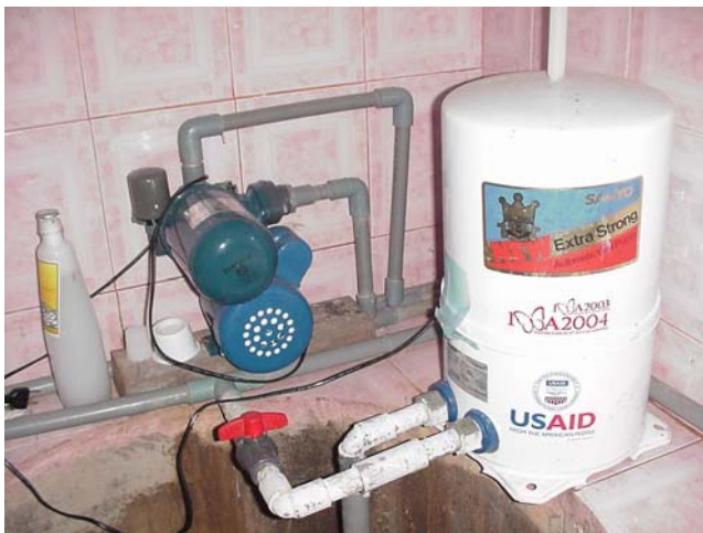
OIG photograph of a USAID-funded pump system provided to a village health clinic in Desa Mibo, Banda Aceh District (Aceh Province, Indonesia, February 2006)
