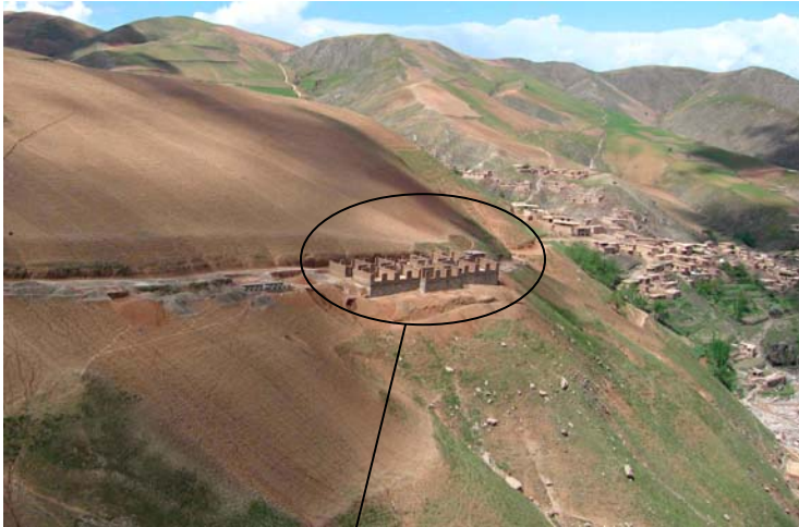
U.S. Army Corps of Engineers photographs of the incomplete Argo Primary School built on the slope of a mountain in Badakhshan, Afghanistan. (May 2006)
