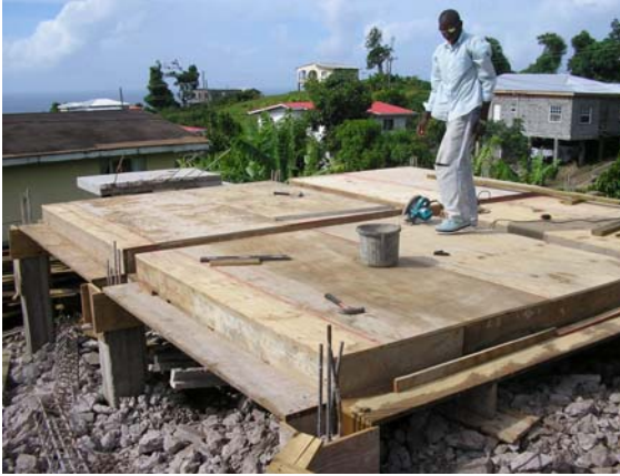
Photo taken by an OIG auditor on January 16, 2006 of a new house under construction in Grenada financed by USAID/Jamaica.
