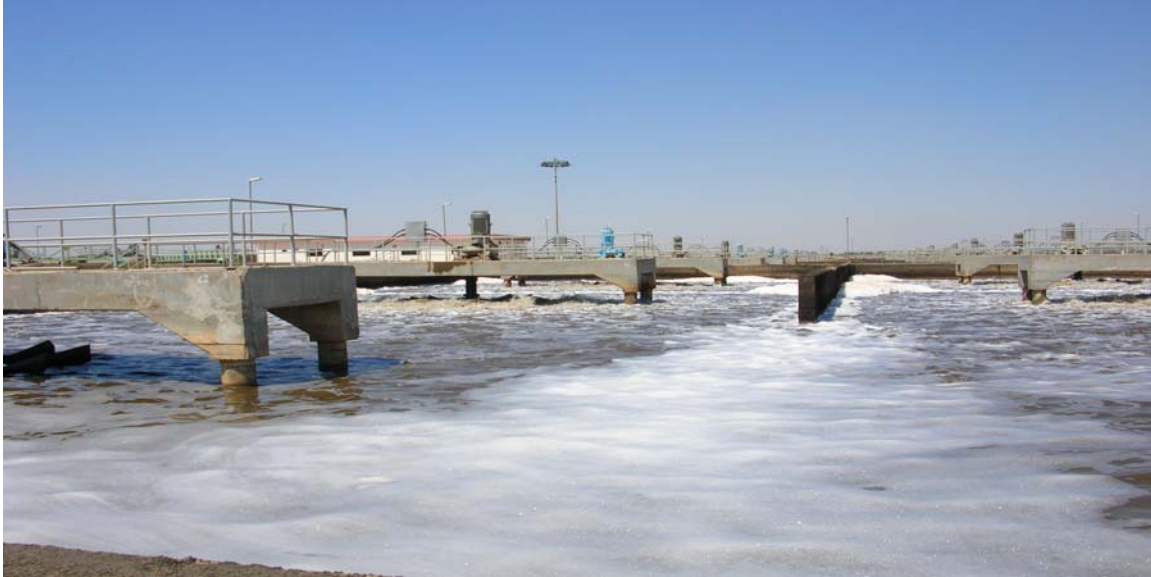
Photograph of one of the eight rehabilitated aeration tanks in operation at the Rustimiyah North Wastewater Treatment Plant funded under USAID/Iraq's Iraq Infrastructure Reconstruction Program. (Baghdad, Iraq; April 2005)
