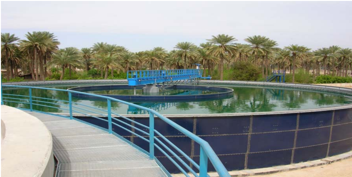
Photograph of one of the six new clarifiers installed at the Shark Dijlah Water Treatment Plant under USAID/Iraq's Iraq Infrastructure Reconstruction Program. (Baghdad, Iraq; March 2005)
