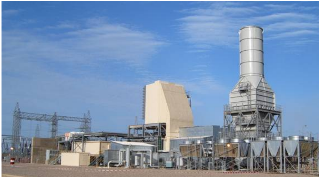
Photo showing the new V64 turbine unit installed by Bechtel at an electrical substation located outside of Kirkuk in northern Iraq. The unit was installed in early February 2005 and added 65 MW to the national grid. (Furnished by USACE; Kirkuk, Iraq; April 2005)
