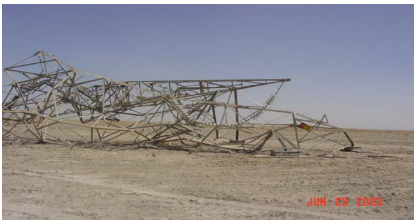
Photograph showing one of the 155 severely damaged transmission line towers along the Khor Al Zubayer-Nassiriyah corridor. USAID funded a project to refurbish these towers to permit the transmission of electricity through this corridor. (Photo furnished by Bechtel; undisclosed location in Southern Iraq; June 2003)
