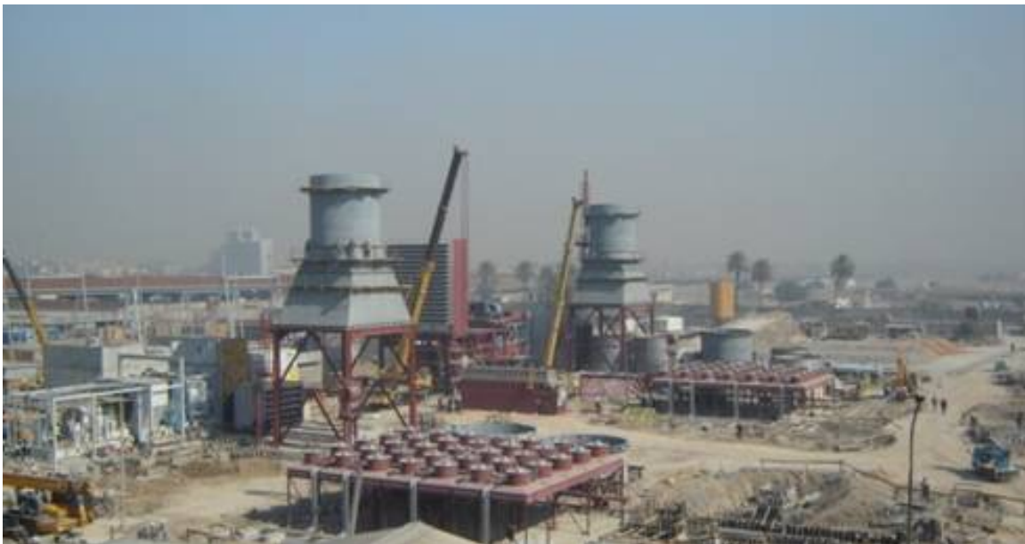
Photograph showing the construction of two new 108-megawatt turbine generators at the Baghdad South Power Plant. This is one of several power-generation projects that are expected to be completed during the second half of 2005. (Baghdad, Iraq; February 2005)
