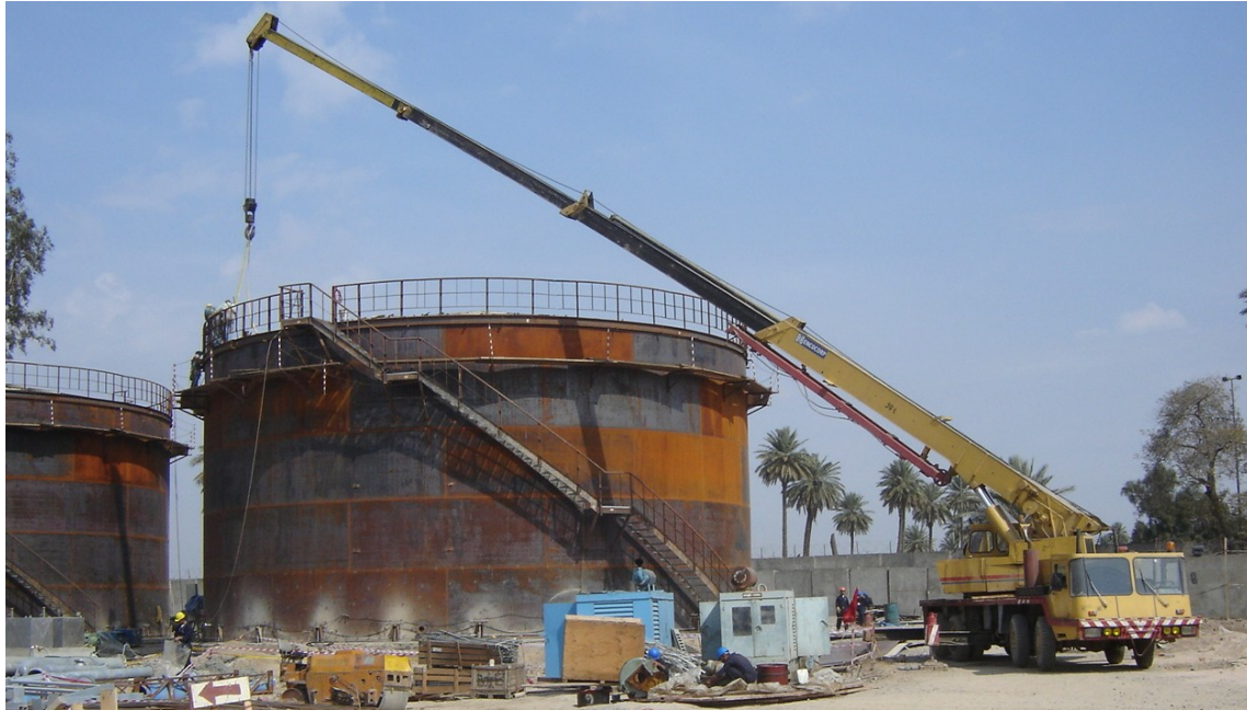
Photograph of fuel tanks under construction at the Baghdad South Power Plant. These tanks will be used to store fuel oil used to operate the power plant's new turbines which USAID was installing under a $163.7 million project. (Baghdad, Iraq; March 2005)
