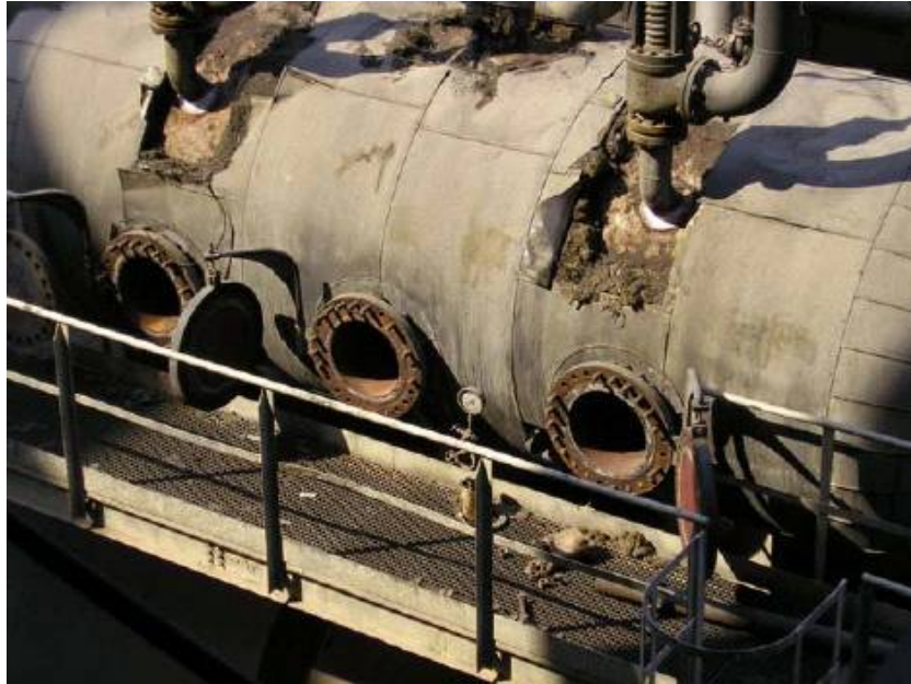
Photo showing the deteriorating condition of existing equipment at the Bayji Power Plant (Furnished by USACE; Bayji, Iraq; September 2004)
