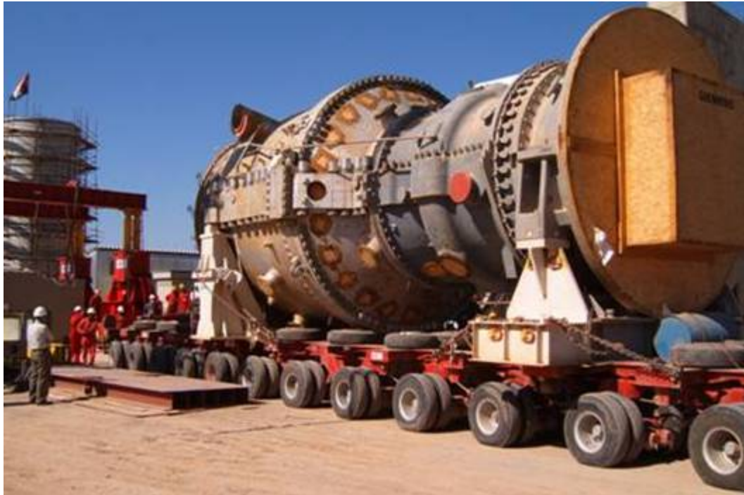
Photograph of the large V94 turbine generator after its arrival at a substation near Kirkuk. Upon its installation in the fall of 2005, the unit is expected to generate an additional 260 MW of electricity for the national grid. (Furnished by USACE; Kirkuk, Iraq; April 2005)
