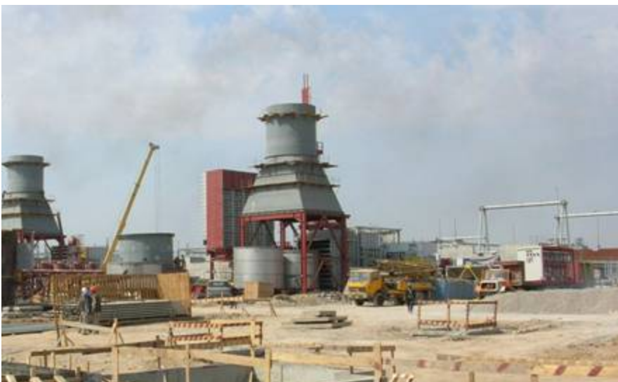
Photograph of new smokestacks under construction at the Baghdad South Power Plant where USAID was funding a $163.7 million power-generation project to install two new 108-megawatt turbines. The project, however, was found to be one of seven that was not achieving its intended outputs. (Baghdad, Iraq; March 2005)
