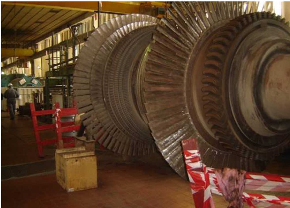
Photograph showing one of the two turbines that Bechtel National, Inc. was refurbishing at the Doura Power Plant in Baghdad (Baghdad, Iraq; March 2005)
