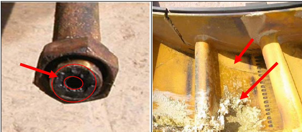
(Left): Photo showing sludge buildup resulting from poor fuel treatment in a fuel line leading to one of the turbines at the Al Qudas Power Plant; (Right): Photo showing a crack and crude oil deposits accumulating inside the turbine. (Furnished by USACE; Al Qudas, Iraq; April 2005)
