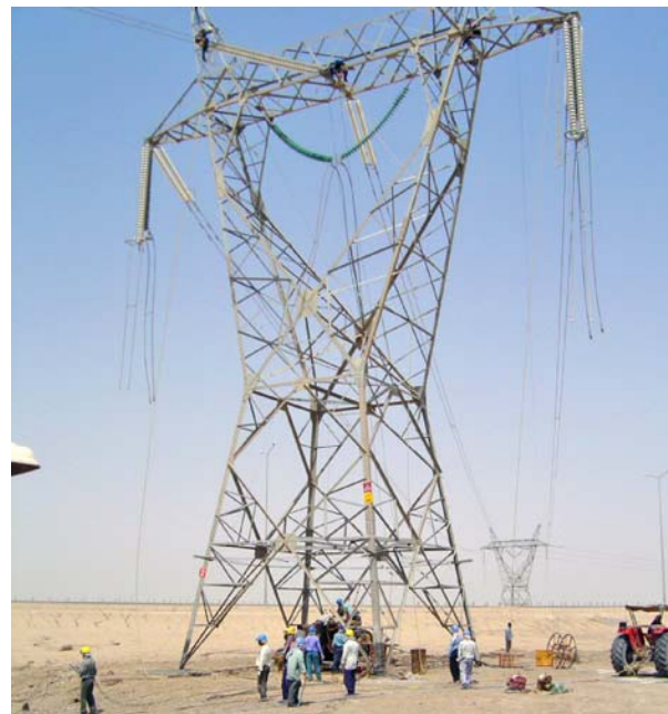
Photograph of one of the towers erected under USAID’s transmission line project (JO-04-004) along the Khor Al Zubayer-Nassiriyah corridor in Southern Iraq. (Photo furnished by Bechtel; undisclosed location in Southern Iraq; undated)
