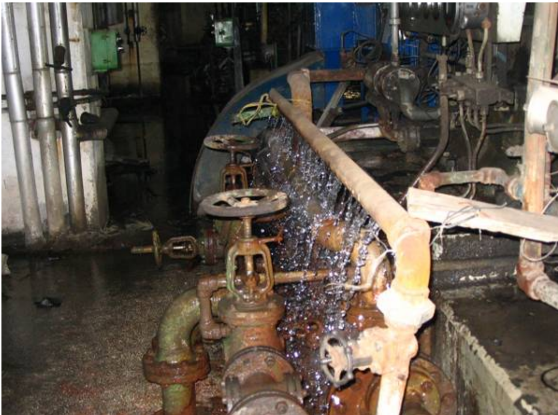
Photograph of water leaking from pipes connected to a feeder pump supporting one of the boilers at the Doura Thermal Power Plant. ME plant staff had performed maintenance work on the pump to repair the leak several months earlier but failed to adequately address the problem. (Baghdad, Iraq; May 2005)
