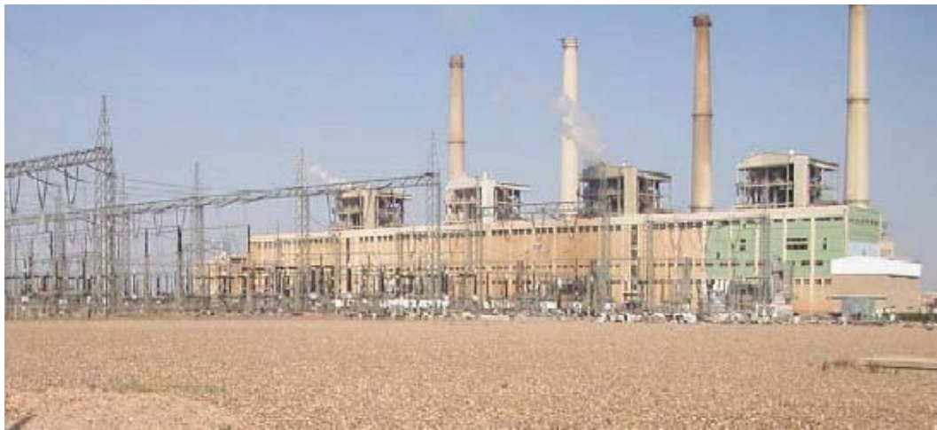
Photograph showing the Mussayab Power Plant where USAID funded a project providing technical and management support to plant staff. The project was terminated in March 2005 due partly to a lack of cooperation from the ME staff. (Mussayab, Iraq; March 2004)
