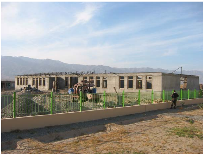
Photograph of the construction of an eight-classroom school taken on October 14, 2004 at Karabagh, Province of Kabul.
