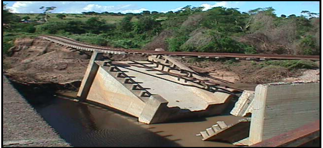
Photograph showing damage to the Limpopo Rail Line at Macarretane caused by flooding in 2000. (Photo courtesy of USAID/Mozambique.)
