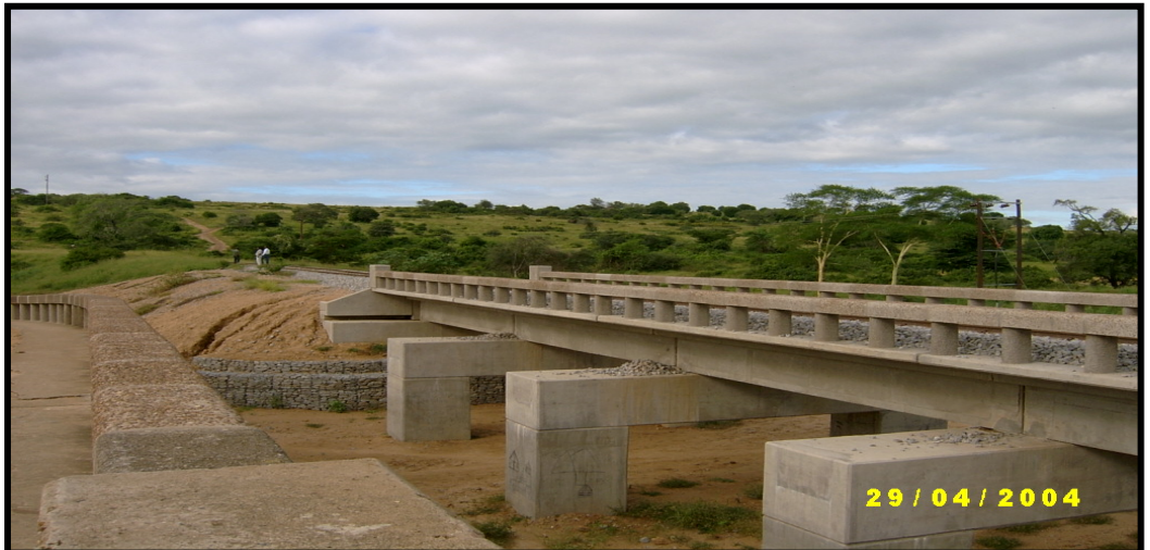
Photograph showing the same portion of the Limpopo Rail Line supported by the reconstructed bridge in 2004. (Photo courtesy of USAID/Mozambique.)
