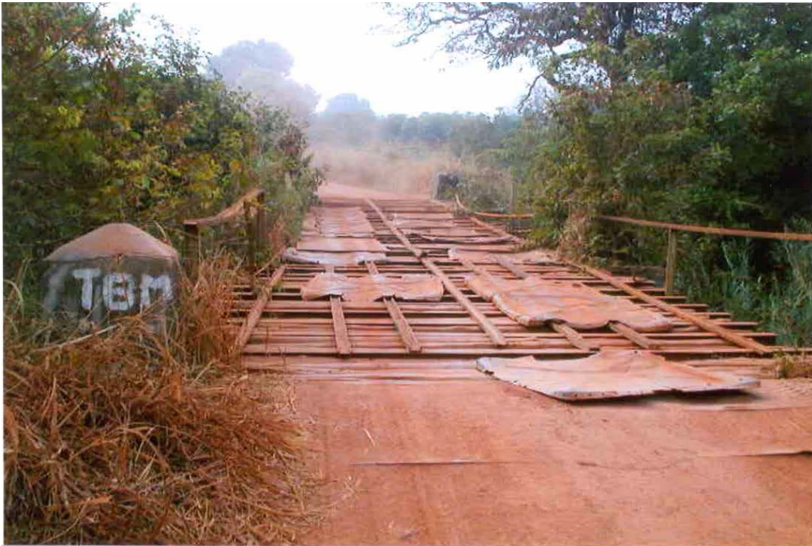
Photograph of makeshift improvements to a road bridge located between the cities of Maridi and Yei, Sudan. (January 2005)
