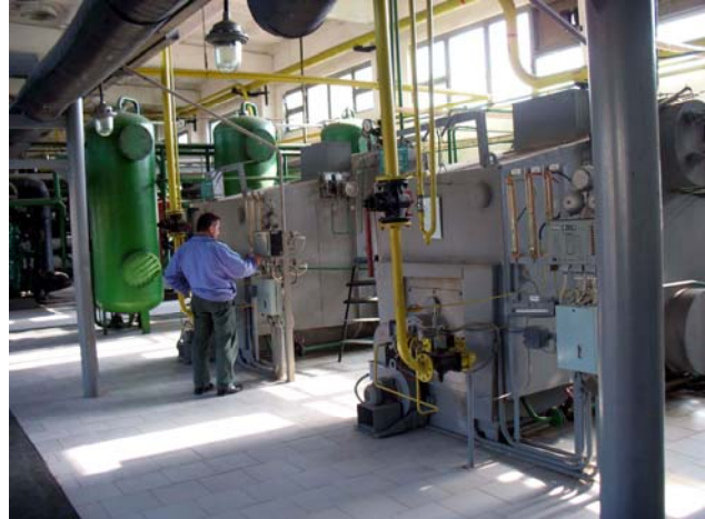
A Combined Heat & Power (CHP) facility in the city of Ivano-Frankivsk, Ukraine.
