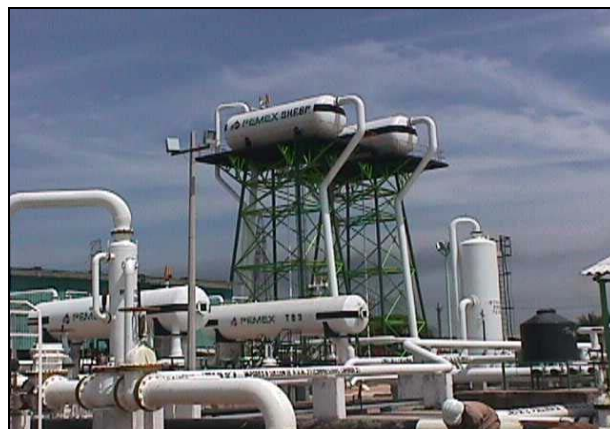
Elevated oil storage tanks and bank of compressors at PEMEX Natural Gas Processor Center
