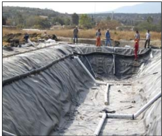
Construction of a pilot biodigester in a small swine farm in central Mexico
