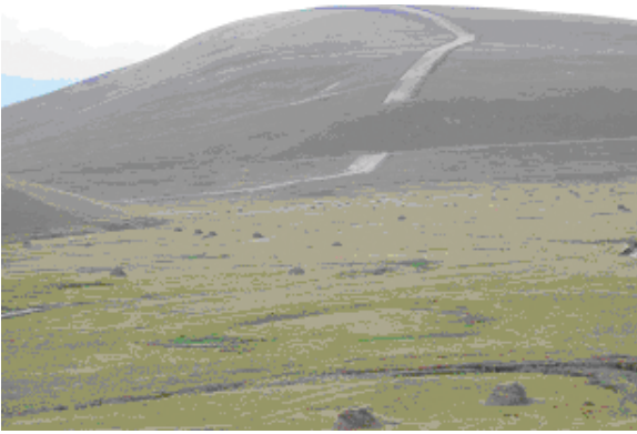
Access road for construction through Qtsia Tabatskuri wetlands. This is an important area for migratory birds, as well as the globally threatened endemic Black Grouse.
