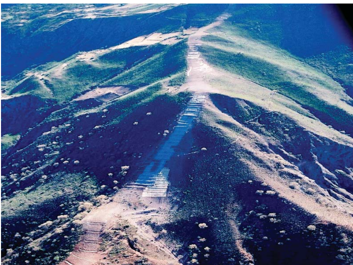
Section of ROW which highlights the use of erosion control barriers, geotech mats and erosion on the side slope.
