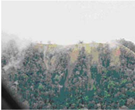
ROW with side slope erosion with some use of geotech mats.
