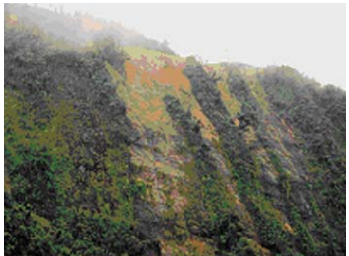
Steep side slope off ROW where no erosion control measures are in place.
