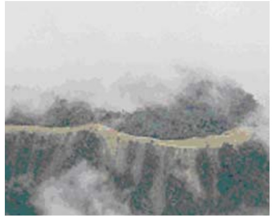
ROW with side slope erosion and absence of erosion control measures on slopes.
