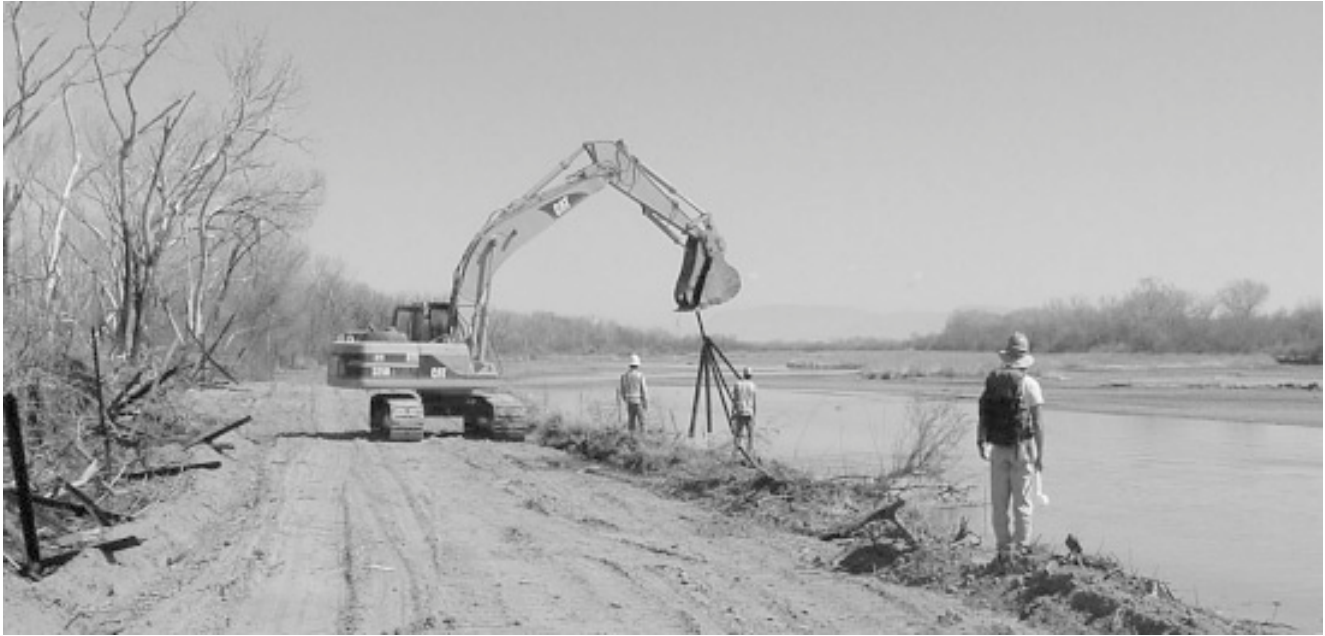
Figure 12. Removing buried jetty jacks at the Los Lunas Rehabilitation Project site. (Photo courtesy U.S. Army Corps of Engineers)
