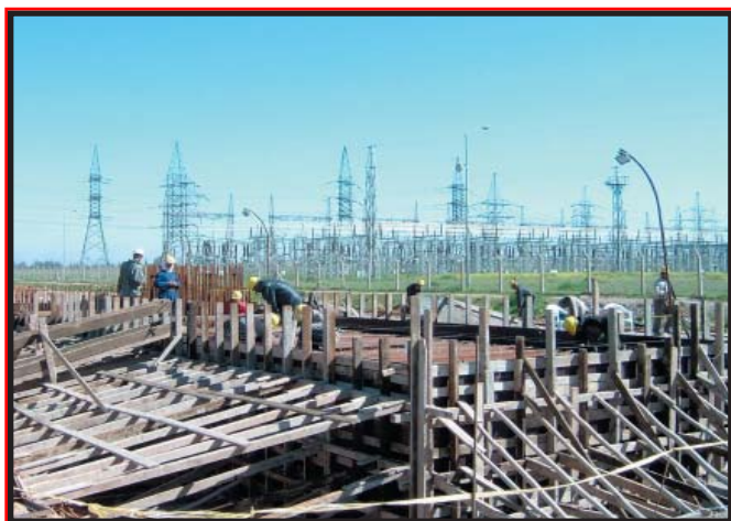
Photograph of site preparation for an electric generation plant in Kirkuk, Iraq.
