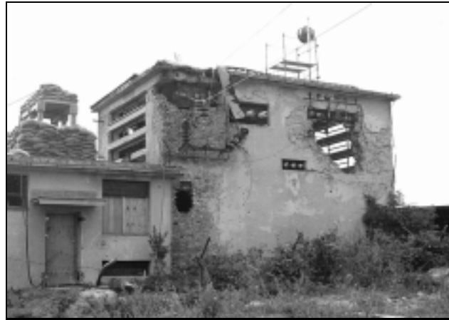
Figure 4 The old Kalesija electrical substation, rebuilt under the MISP.
