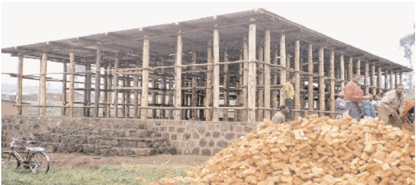
Construction of a warehouse for storing seeds in Ruhengeri District, Rwanda was financed with funds generated under the emergency food sale program.
