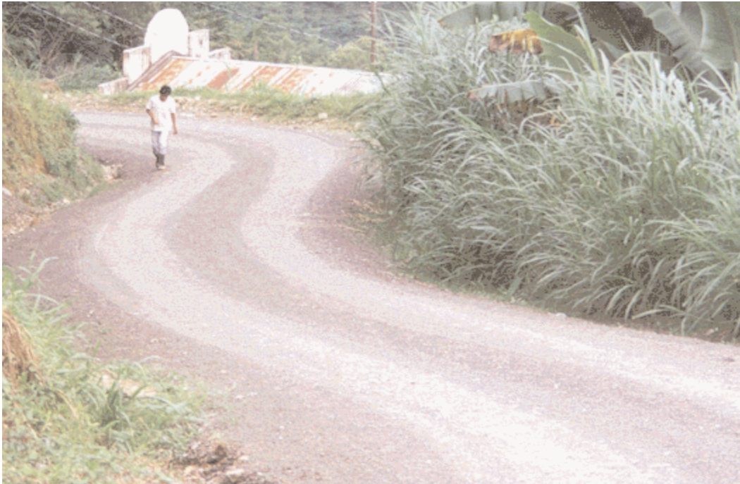
Rural road reconstructed by the National Coffee Association as part of USAID/Guatemala's roads and bridges reconstruction activity, Alta Verapaz, Guatemala
