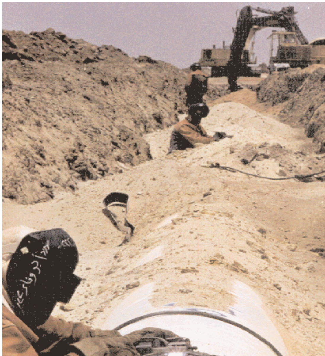
Welders complete a piping segment of the wastewater treatment project in Egypt.
