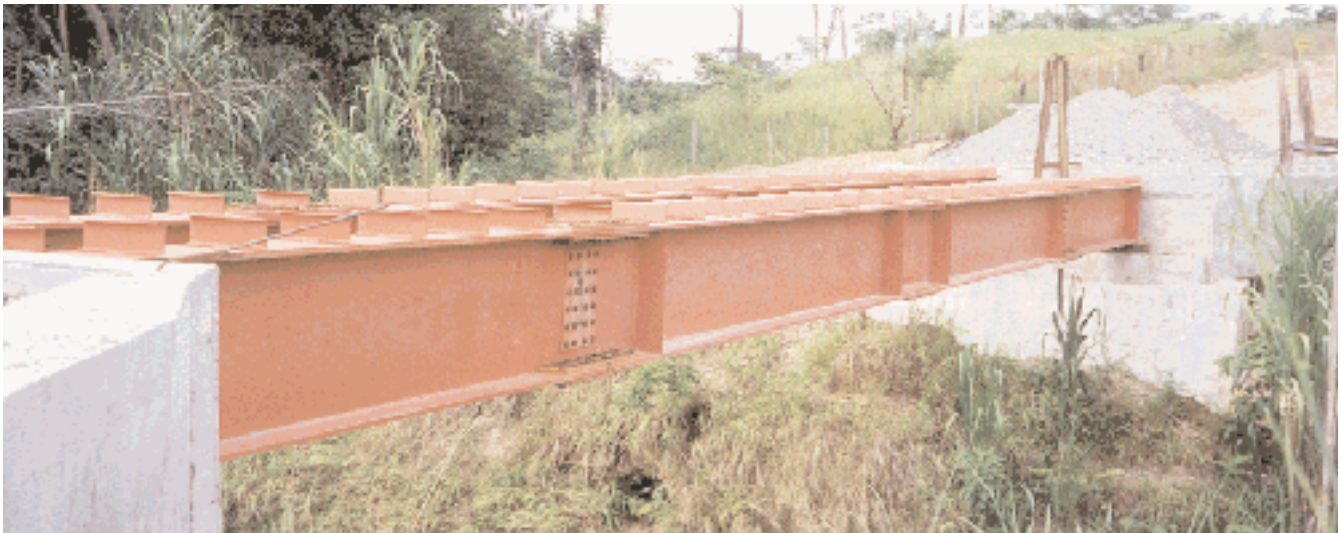
Santo Tomas Bridge construction project managed by the Cooperative Housing Foundation, Ixcán, Guatemala
