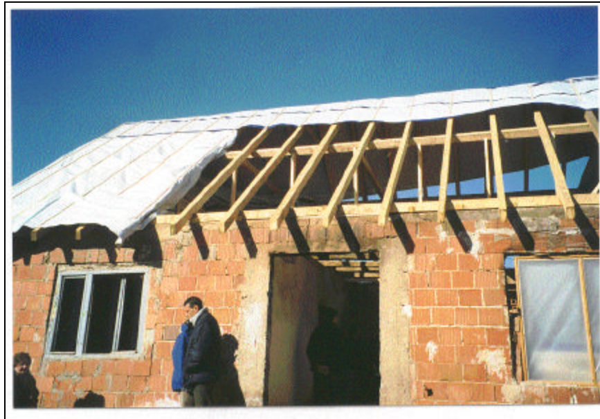
A typical home in the Podujeve, Kosovo is being repaired with material provided by USAID/OFDA through its partner, World Vision International
