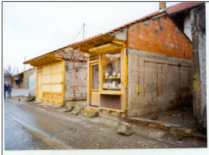
Owners repaired these shops. Thirty-nine others will be reconstructed under the USAID/OTI project and will look similar. The jewelry store on right is open for business.
