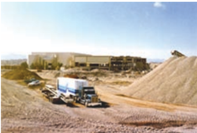
Figure 8. On-site recycling of demolition debris for use as aggregate at the former Cinderella City shopping mall in Denver, Colo.
