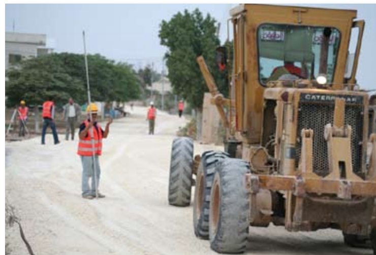
A Palestinian surveyor helps build a road in the West Bank city of Jericho, the lowest city on earth and one of its oldest. USAID is building 10 kilometers of roads in the city.
