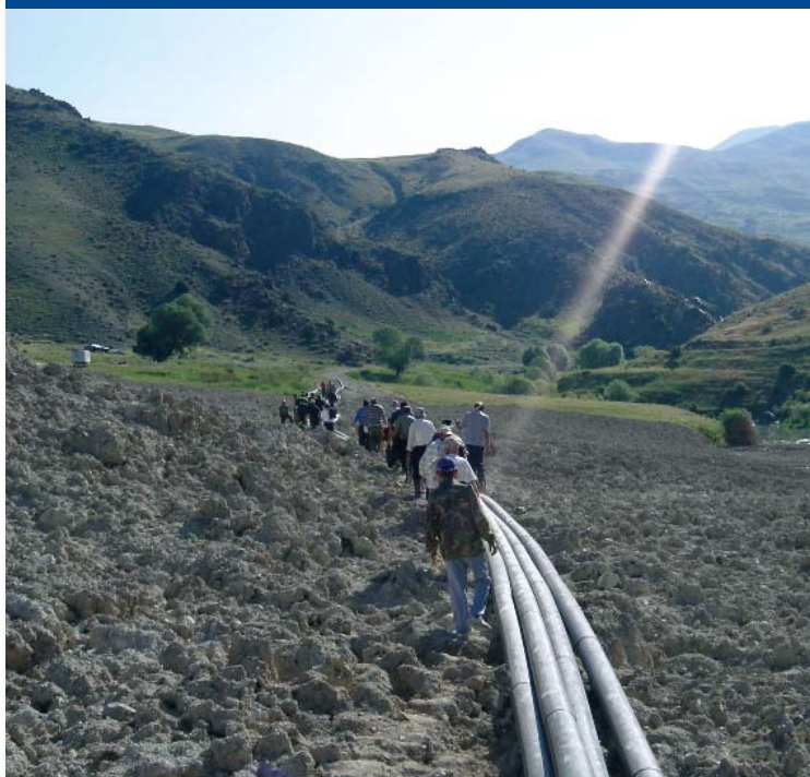
Workers install new potable water pipes for the Jermanis-Vedi pipeline in Ararat Valley, Armenia.
