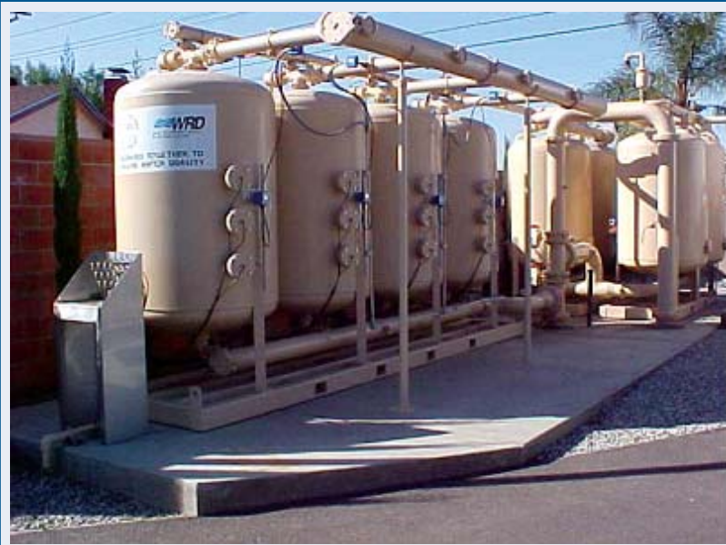
Many water sources in the nation have arsenic levels above the future regulatory limit of 0.010 milligrams per liter (mg/L). To meet the more stringent arsenic regulation, the pilot plant shown is examining adsorptive and specialty media for optimal arsenic removal.
