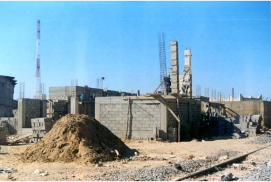
Construction of Dokrarat wastewater treatment facility for tannery effluent: the chromium recycling plant.
