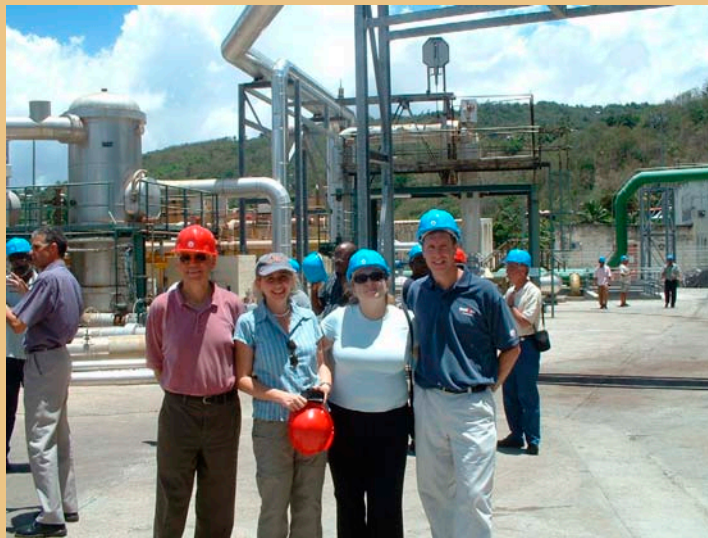
The Bouillante geothermal power plant in Guadeloupe – part of the Eastern Caribbean Geothermal Development Project that covers Saint Lucia, Saint Kitts and Nevis, and Dominica.
