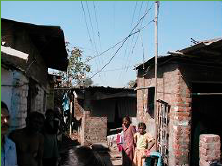
Illegal electric connections.
