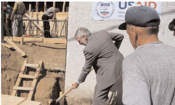
Dr. Michael Farbman, USAID/Kosovo Director laying foundations of the annex to the Public Library in north Mitrovica.
