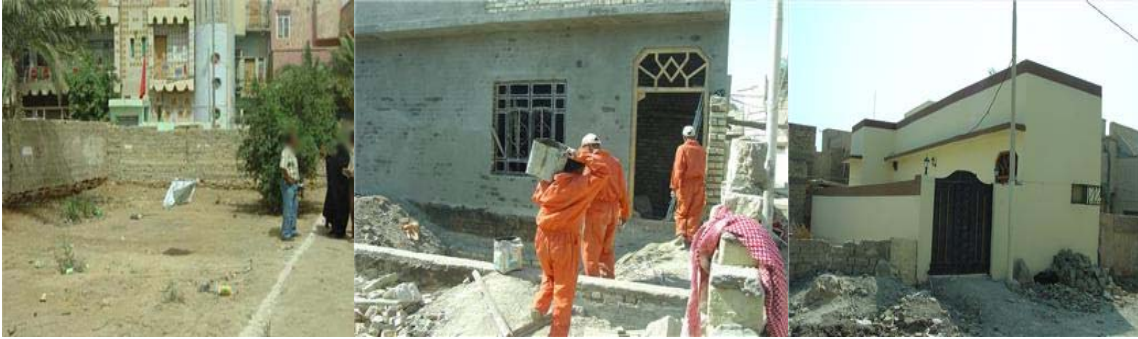
Figure 3. Photos of a Marla Fund project to reconstruct the home of an Iraqi family after it was destroyed as a direct result of Coalition Forces military operations. Source: USAID/Iraq
