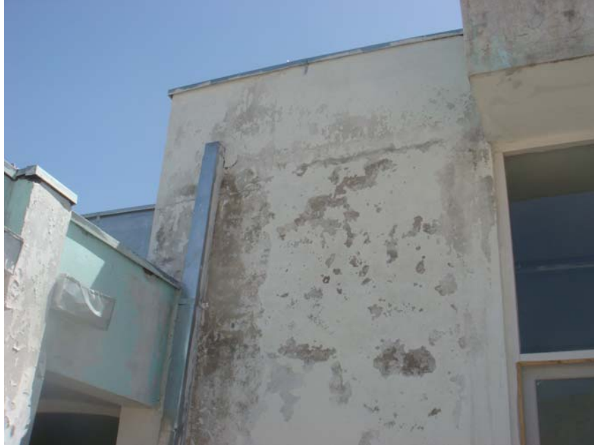
Photograph of a building constructed in Parawan Province, displaying the incomplete exterior and surfacing work. (Office of Inspector General, April 2008)
