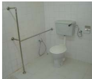
Toilets in Nakulugamuwa
