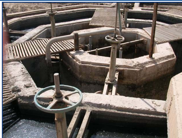
Above: Baghdad's three sewage plants are inoperable. USAID Photo
