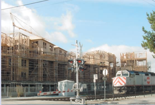
Construction underway on Phase I of the Franklin Street project, which will provide 206 residential units at the Redwood City Caltrain Station.
