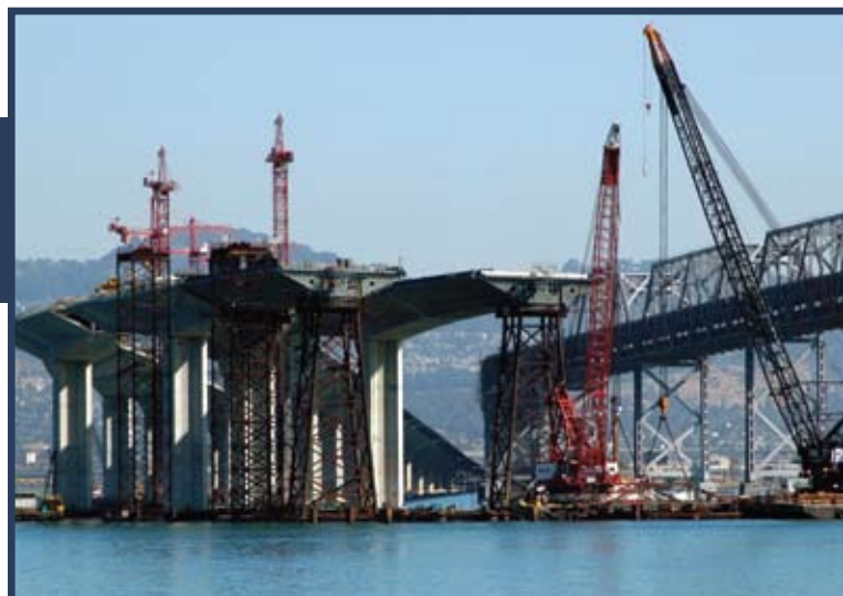
Construction of the new Bay Bridge in California involves use of recycled fly ash.
