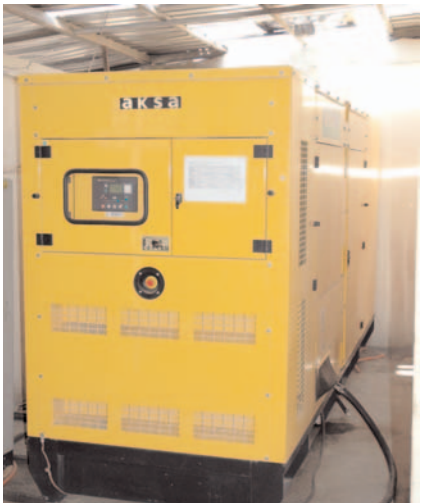
(top) control panel to monitor system, (middle) three stage fuel filter for generator, (bottom) Reliable power is one of the key elements in maintaining sensitive IT and communications equipment.
