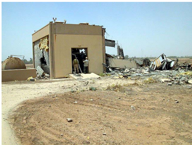
Destroyed Airfield Lighting Substation
