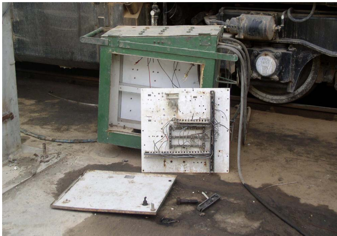
Figure 8. Al Basrah shed jacking control panel
