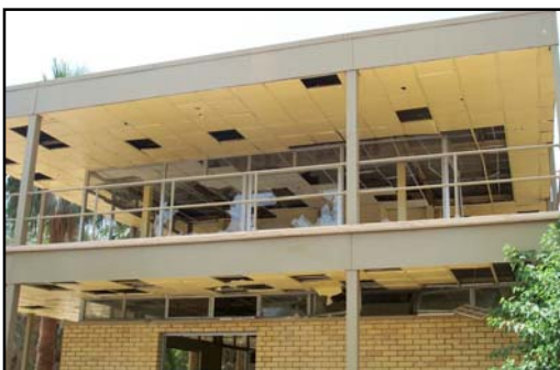
Figure 25 Many buildings require only aesthetic repairs.
