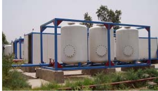
Typical compact water treatment unit
