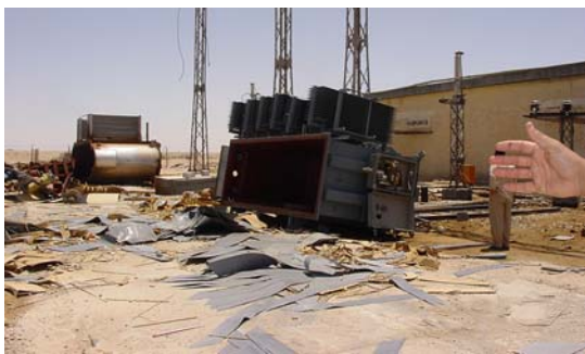
Rumaila Oilfield Substation Transformer Destruction
