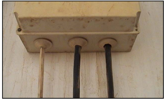
Figure 17 Temporary glands to be replaced with permanent, rodent-resistant, IP 54 (minimum) international standard glands.
