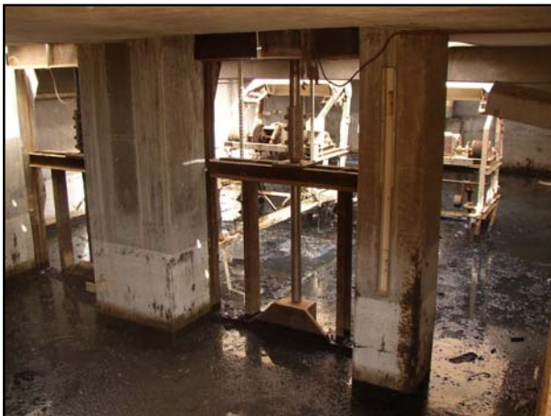
Figure 29 Penstocks shown in Figure 29 require rehabilitation due to lack of maintenance.
