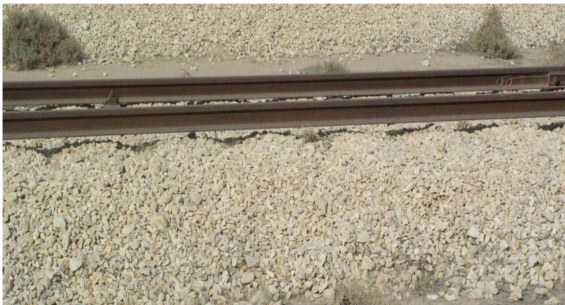
Figure 5. Unsupported Rail. While this is one of the few locations with ballast, the sleepers (ties) have been stolen, making the line unusable.
