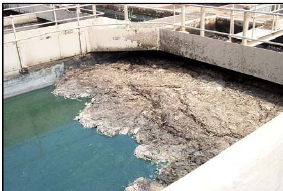
Figure 31 Photo of an aeration tank with old sludge decaying on cleaning will be required prior to refurbishment.
