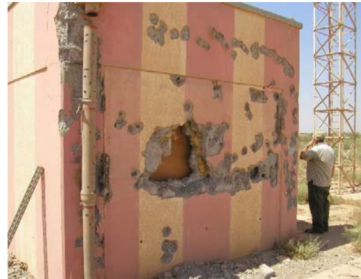
Damaged Airfield Building
