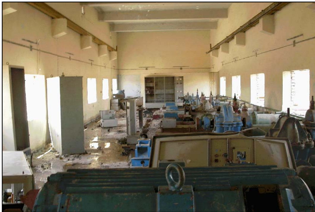
Figure 15 At many plants, the power cables, signal cables, and pump control instrumentation has been removed.
