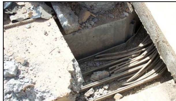
Figure 24 Concrete cable troughs exposing power cables beneath the broken lids create a potential hazard and provide rodents with a man-made habitat.
