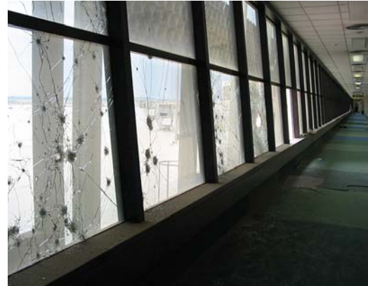
Damaged Terminal Windows – Baghdad International Airport
