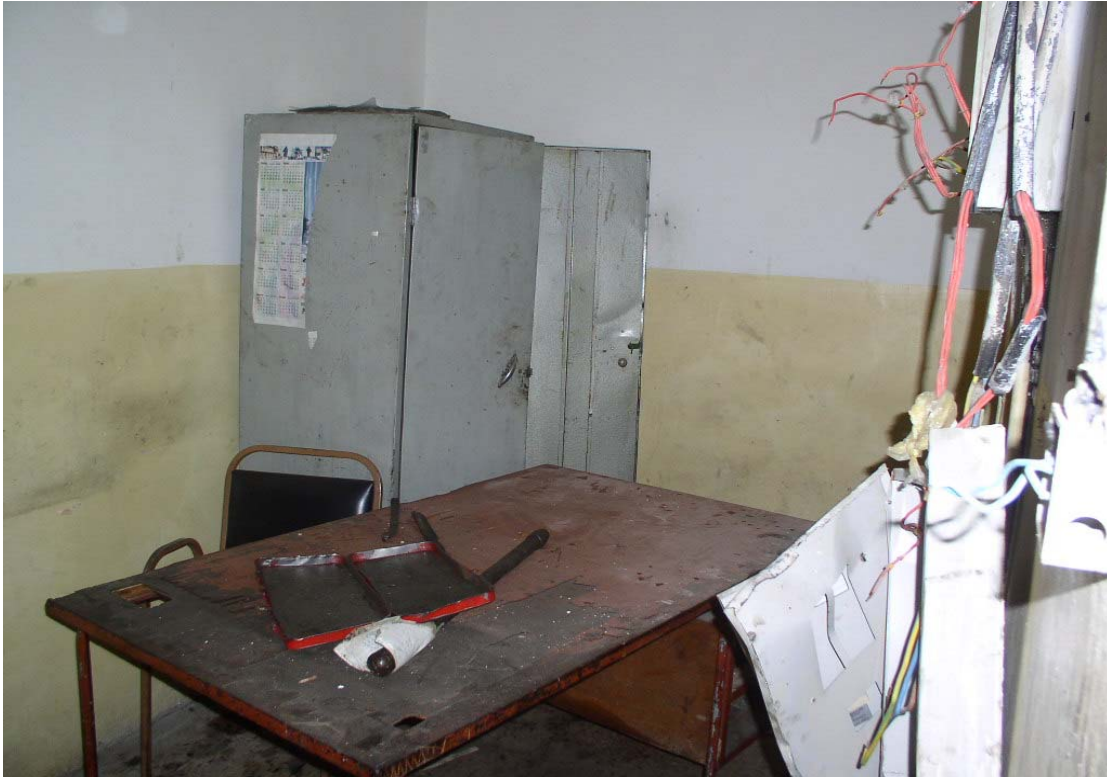
Figure 10. Typical wiring condition in Al Basrah Locomotive Shed
