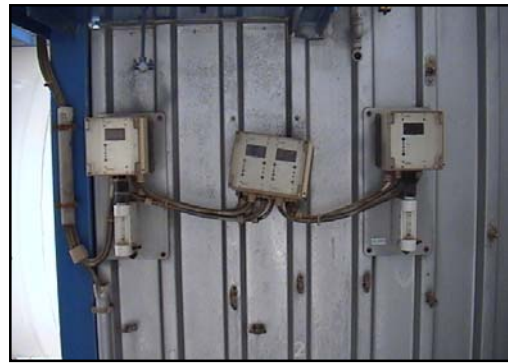
Figure 22 Some equipment is fully operational and requires only minimal work. The unit shown here needs to be mounted in a more appropriate, functional, and safe manner.
