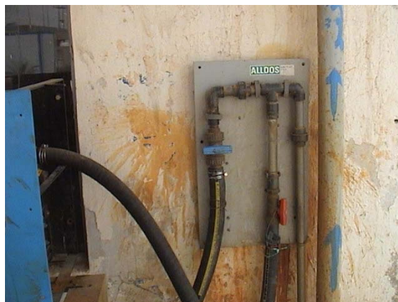
Figure 9 In many cases, the resin inside UPVC fittings has become brittle causing leaks to occur.
