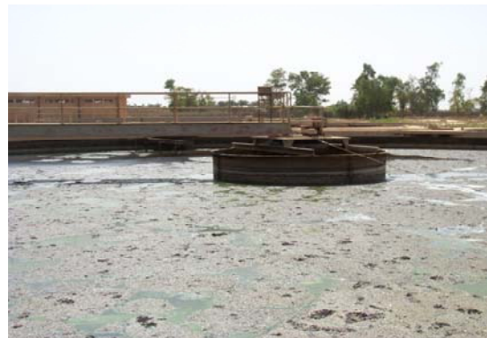
Out of service clarifier
