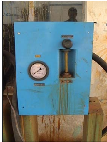
Figure 14 Chlorination equipment failed due to lack of maintenance and the lack of chlorine often caused operators to shutdown the device for long periods of time resulting in blockages.
