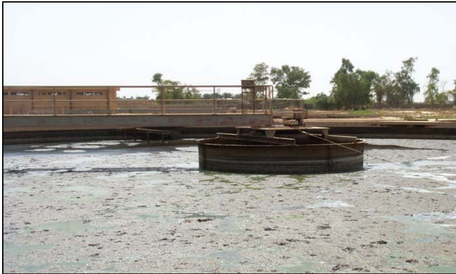
Figure 35 Out of service clarifier.
