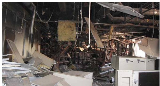
Conflict Damage—Basrah International Airport
