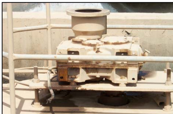
Figure 34 Aerators, gearboxes, and other key mechanical equipment have either been looted or cannibalized for spare parts for other units.
