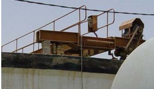
Figure 6 A scraper unit on bricks, a result of looting.
