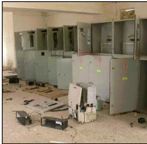
Figure 12 Control panels stripped of contents.
