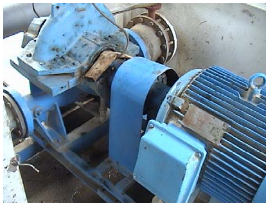
Figure 8 Pumps will require testing under all conditions to ensure availability. Many will require refurbishment rather than replacing.
