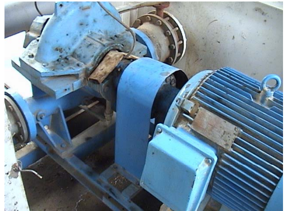
Pumps will require testing under all conditions to ensure availability.
