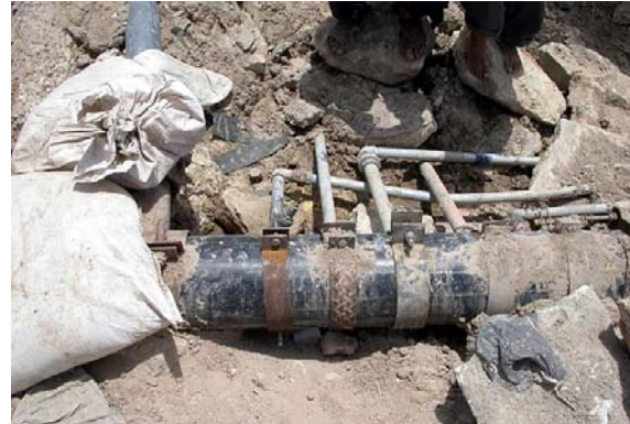
Illegal tapping points on water supply pipe
