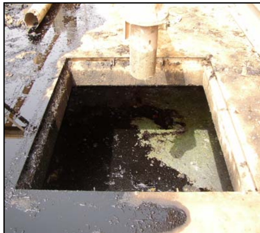
Figure 30 A lack of grease reduced control over the the plant's operation often resulting in flooding
