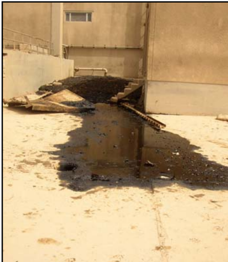
Figure 27 Many containment walls require attention as the load bearings have grown larger than anticipated.
