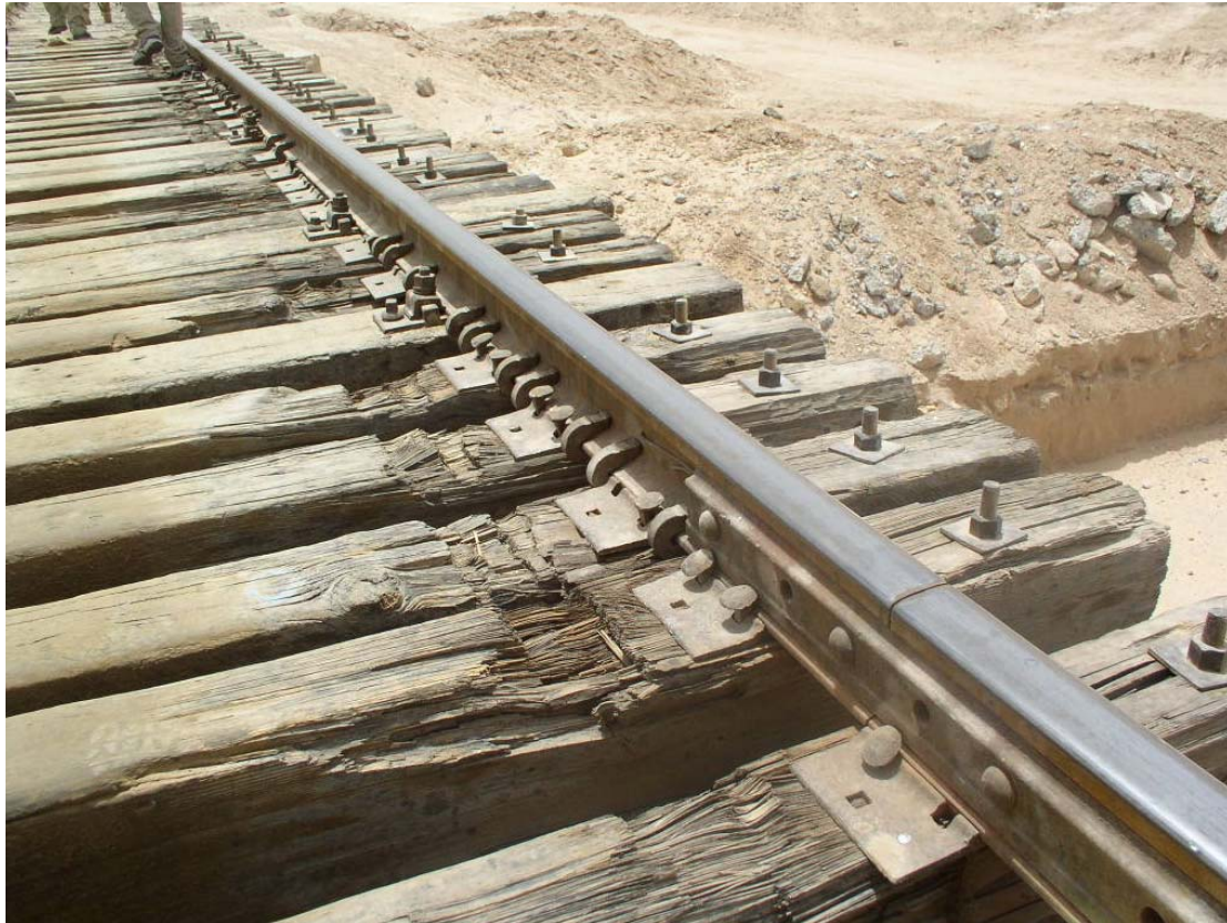
Figure 4. Main line over culvert with evidence of derailment. Note poorly bolted fishplate over the culvert and inadequately secured sleepers.
