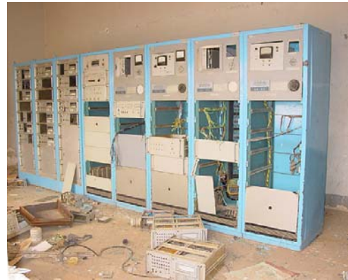
Control System for Substation
