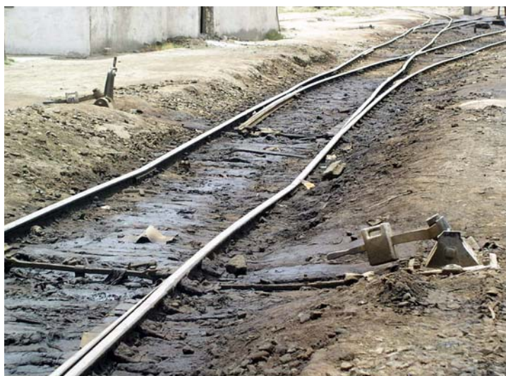
Worn Out Track in Al Basrah Area
