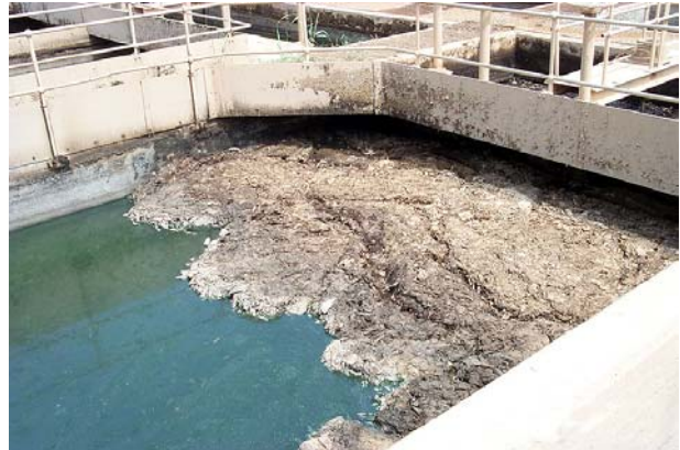
Aeration tank with old sludge decaying at base.
