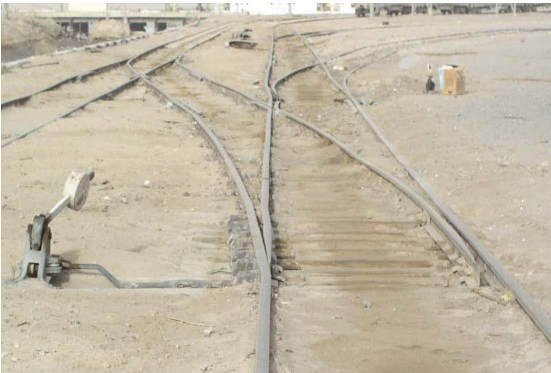
Figure 1. Kinked and sunken track in the old port at Umm Qasr.
