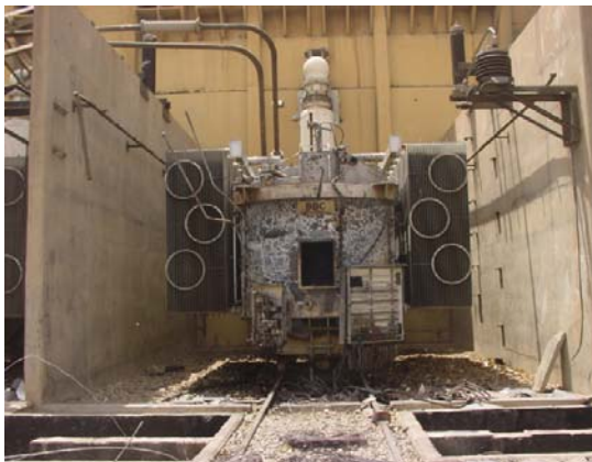
Destroyed Al Qurnah Substation
