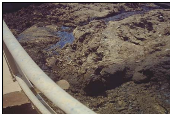
Figure 33 Out-of-service primary clarifier. Sludge crust produced by rising solids provoked by gas production from decaying sludge. Cleaning will be required before refurbishment.
