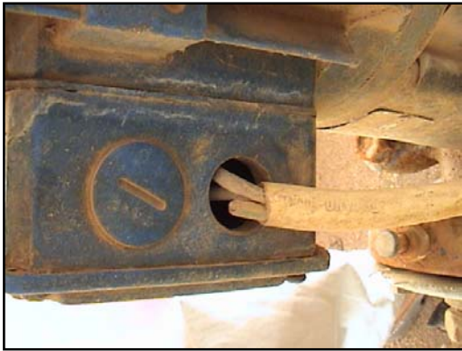
Figure 16 In some instances, where protected cable was not available, the operator has used domestic flexible mains cable without a gland. This example puts the entire site in danger as the cable runs past chlorine tanks.
