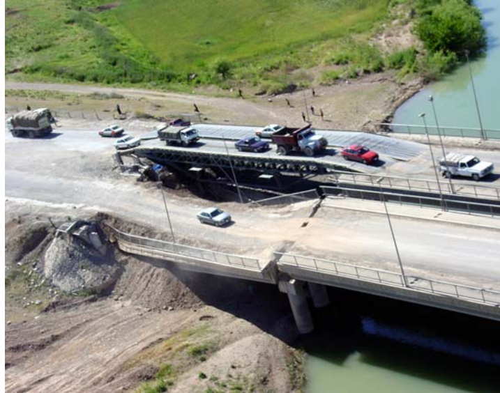
Traffic Still Flows Over Dangerously Damaged Bridges
