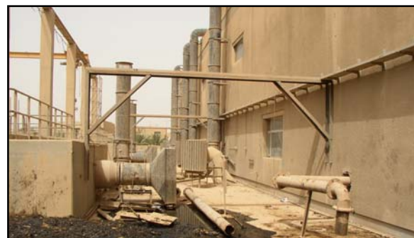
Figure 26 Due to the inoperability of control valves, a cleanup operation will be required at most wastewater treatment plants
