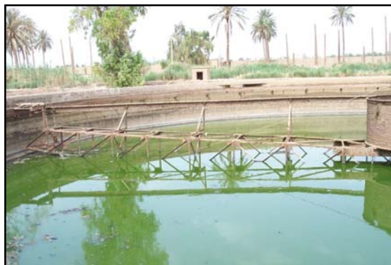
Figure 32 Out-of-service clarifier with old decaying tank base; sludge at base.
