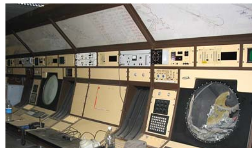
Outdated Radar Equipment
