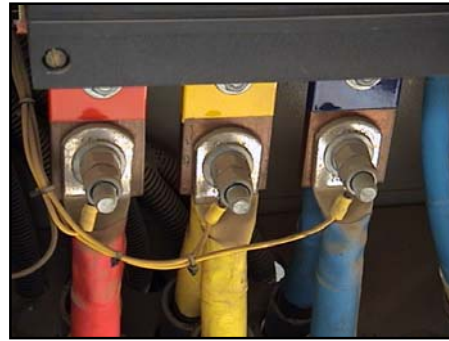
Figure 11 A three-phase supply is available at most sites surveyed, however, in some cases there is no provisions for a backup supply.
