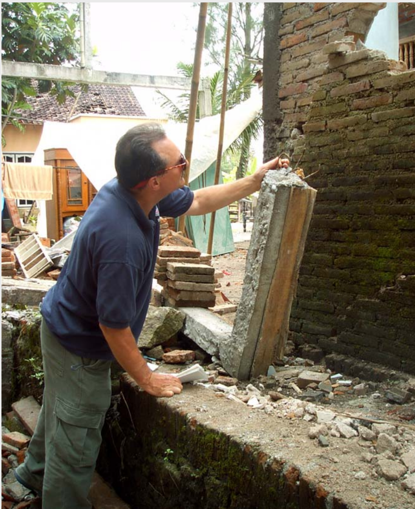
An OFDA shelter specialist examines earthquake-damaged buildings in Indonesia (Alfred Nakatsuma, USAID).
